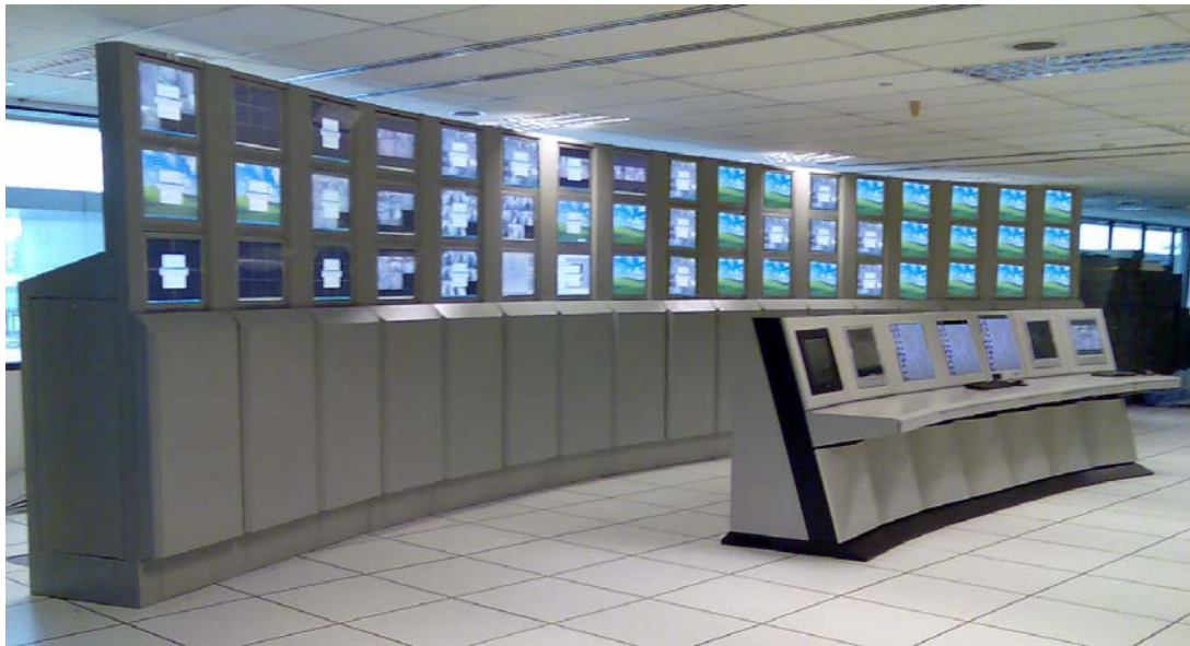
Housing 55 pieces of LCD monitor and equipment inside the Kwik console, this is a typical application in a CCTV control center.
